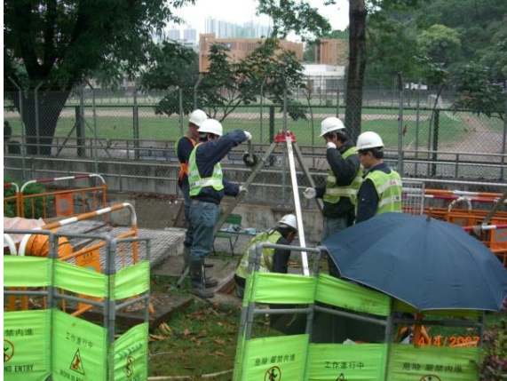
A: Personal protective equipment shall be used when entering the manhole.
