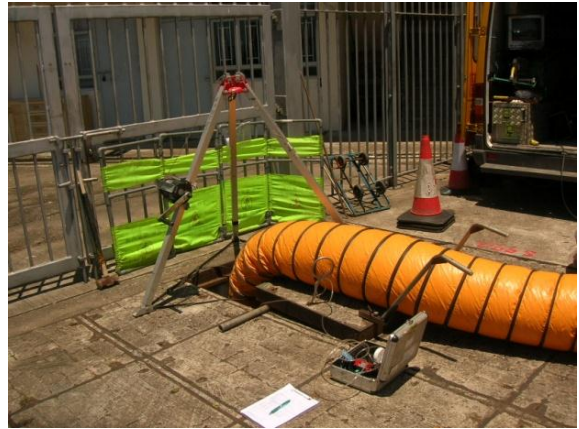
B: The manhole shall be sufficiently ventilated before investigation.
