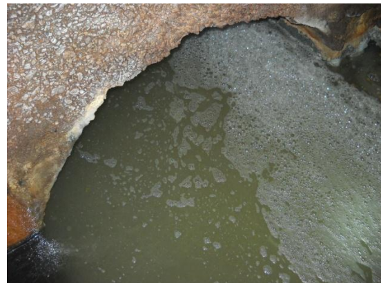
Figure 1.6 Surging Sewer of the City
