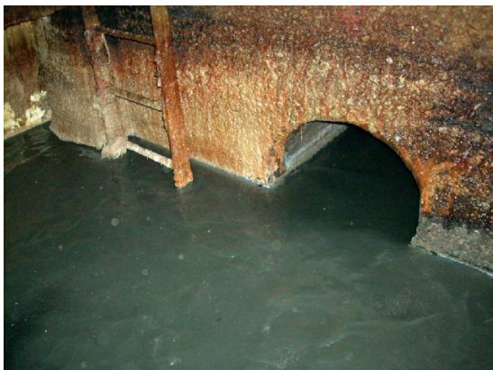
Figure 1.5 Surging Sewer of the City
