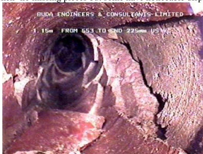
B: Collapse of pipe section with 30% reduction in cross sectional area
