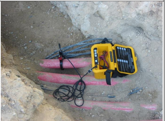
D: A signal clamp is used on an exposed cable duct.
