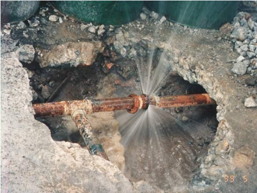
A: Water burst from a deteriorated water main.
