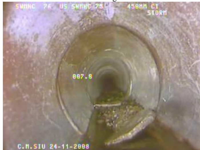
B: Deposit Settled- Coarse material deposits at the bottom of the pipe
