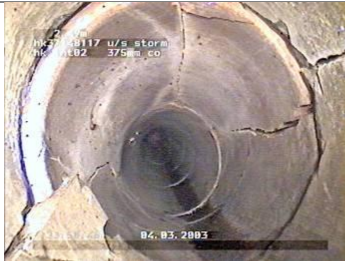
A: Broken- no missing pieces but some have noticeable displacement
