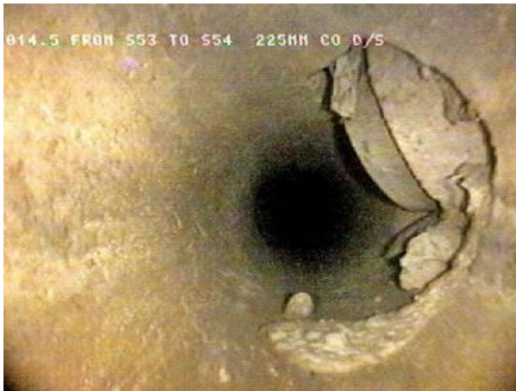
B: Connection Defective- A connection intruding into the main pipe at 2 O'clock
