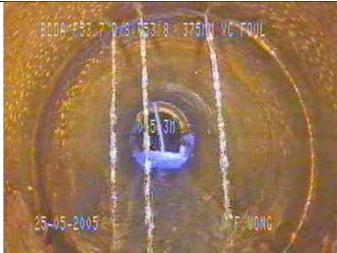
D: Infiltration- Groundwater running continuously through faulty joint
