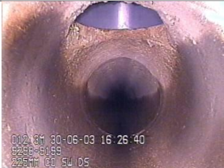
A: Connection- A connection at 12 O'clock with defects and is in service
