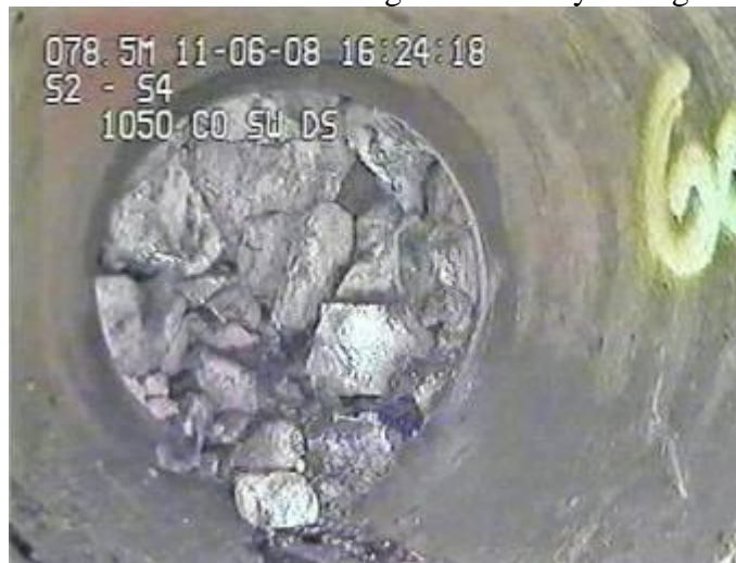
E: Obstruction- Boulders laying in the invert
