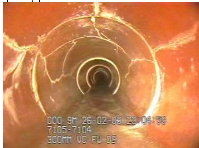
C: Multiple Crack from 9 to 2 O'clock
