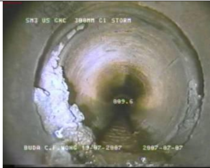
A: Deposit Attached- Foul material from the sewage attached to the inner wall of the pipe
