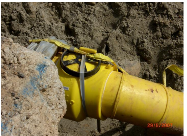
F: A Mini-Marker installed on a gas pipe.
